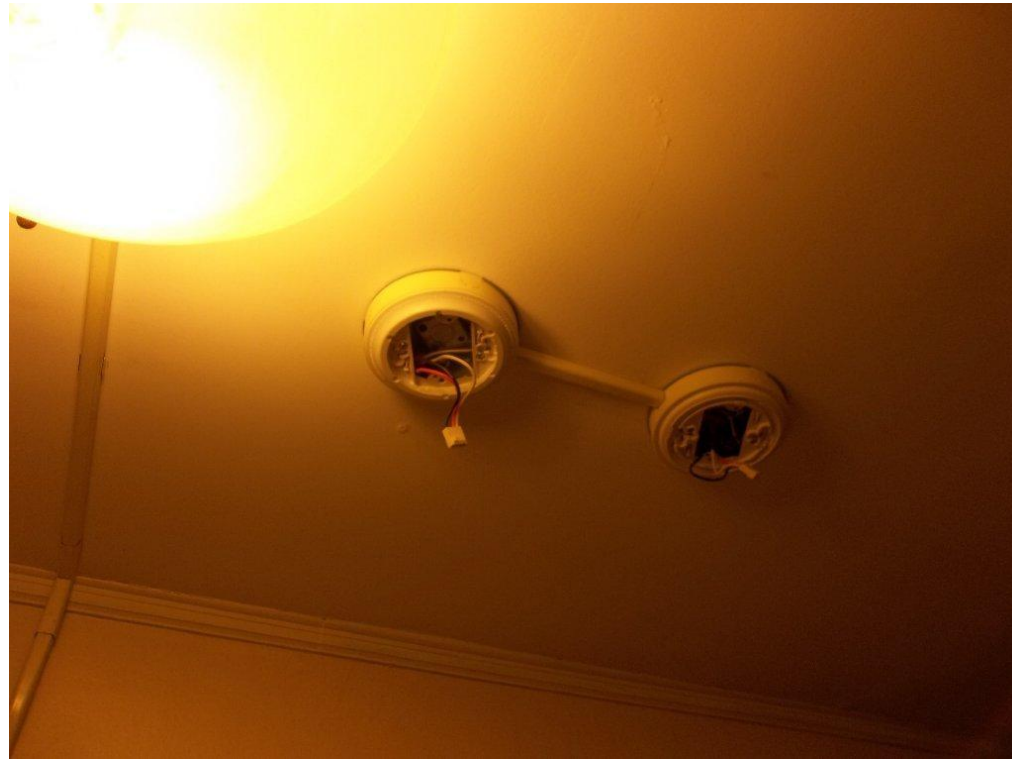
smoke/carbon monoxide detectors removed
