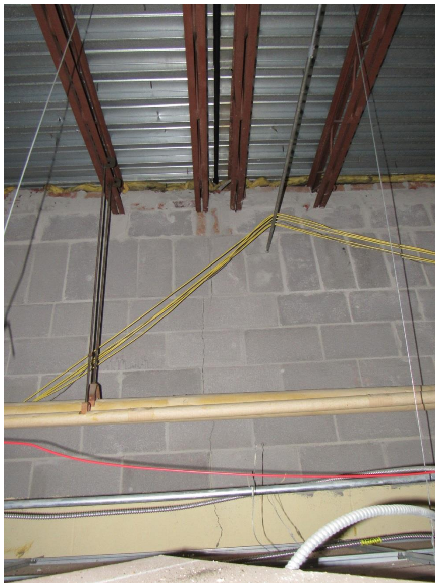
Figure 3 – Crack in CMU wall is cosmetic and not a structural concern.
