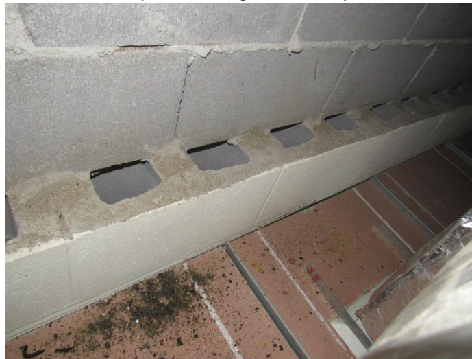
Figure 1 – CMU Walls are ungrouted and unreinforced.
