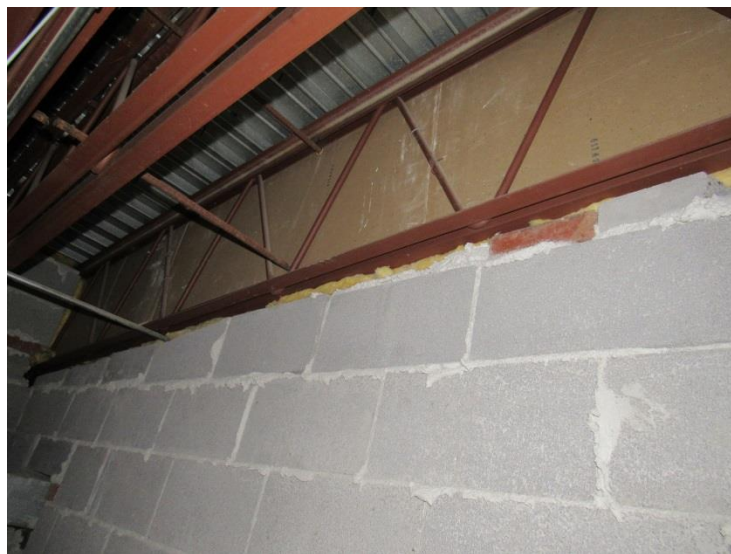
Figure 2 – Gap between top of CMU walls and steel structure
