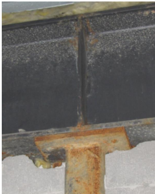
Figure 5 – Bolts Missing in Beam Column connection
