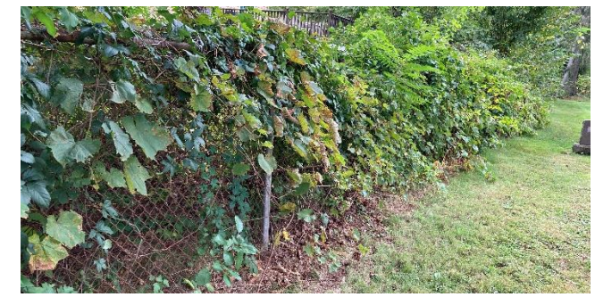
Existing chain link fence to be replaced
